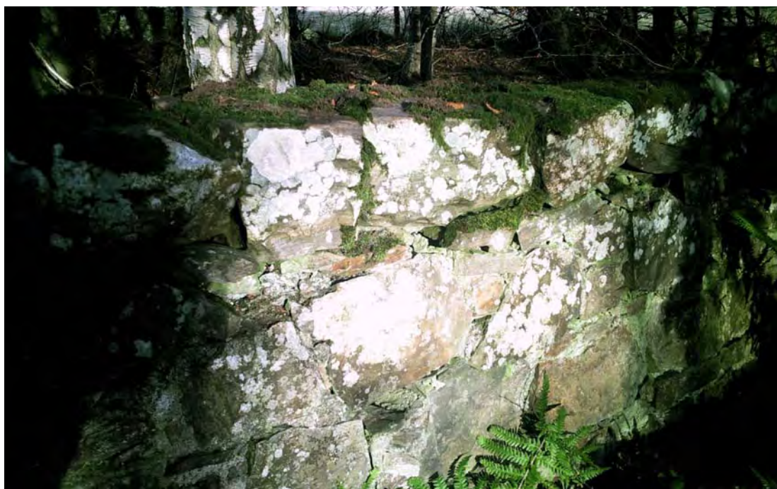
An example of a stone and lime dyke along the avenues at Cobairdy
